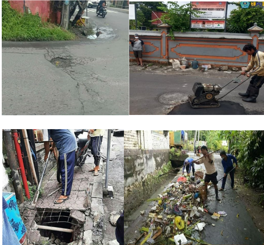
Figure 2: Activities of pavement construction maintenance and drainage of Denpasar city roads during the covid-19 pandemic
